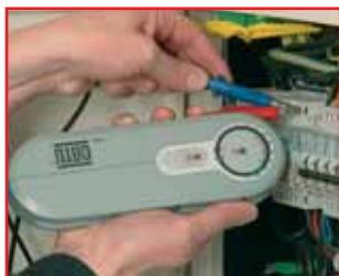
Picture of installation without presence voltage.
